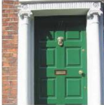
3. Only a small area of the facade is visible. The joints in materials are visible and details are easily read.
